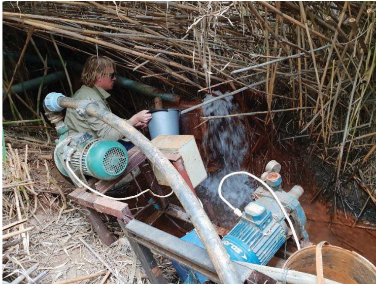
Figure 2-24 Groundwater sampling directly from spring outlet pipe.
